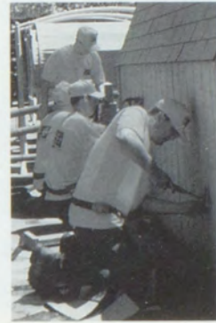
Team members work on the frame of the shed. Eight teams competed in the competition, IHS was honored with placing fourth over all.
