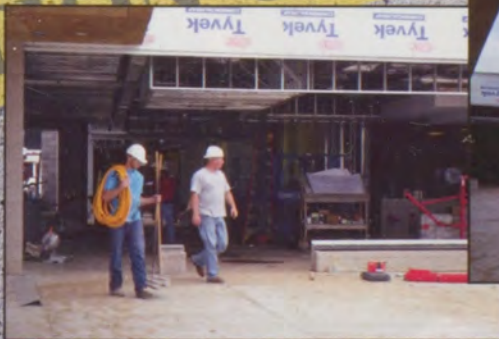
Nabholz employees walk through what will eventually become the new front entrance into IHS.
