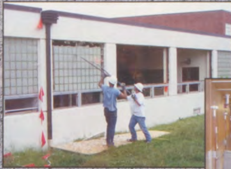
Construction workers knock out glass tiles from classroom windows in the 300 hall.
