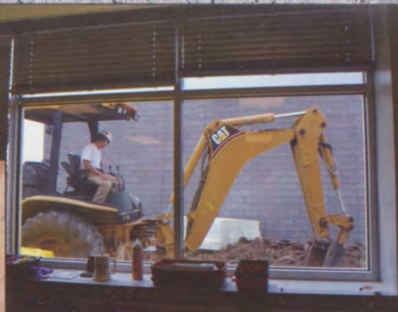
It was common for students to observe ongoing construction. This is the view from Room 311, where dirt work went on with the new gymnasium.
