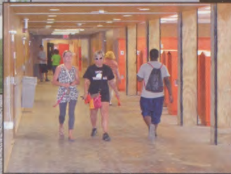
Layne Wilson and Coach Speicher walk through the newly renovated 300 hall, before the columns and flooring were complete.
