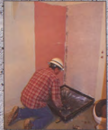
A construction worker removes the shower from one of the old coaches' offices.
