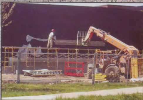
Looking west toward the new performing arts center construction. IHS students went without an auditorium during the 2010-11 year.
